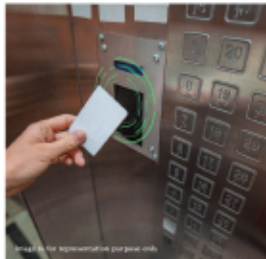
Access controlled Elevators
