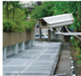
CCTV surveillance in Common Areas
